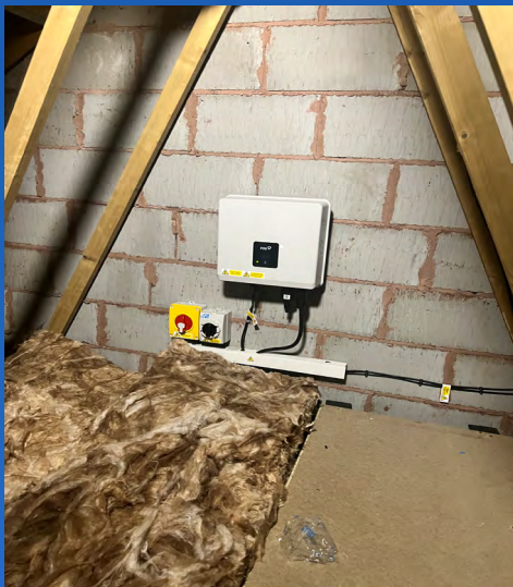
Inverter for solar panel system
