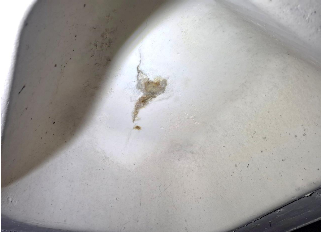
Photograph 02: local staining from corroding reinforcement
