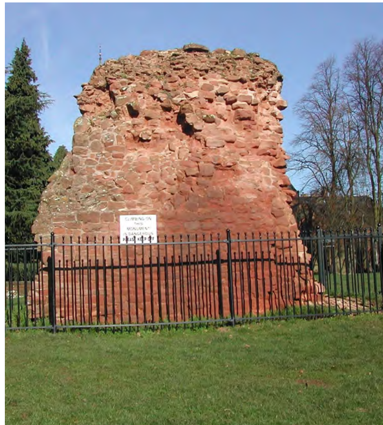
Above: Chapter House wall, south side. The railings were installed as a safety measure in 2003.
