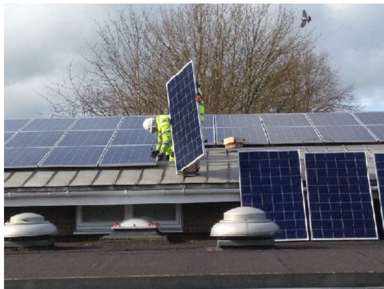
Solar panels for the school
