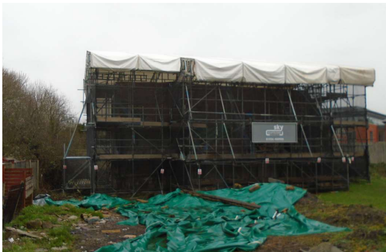
Photo of Master's House c 2020 following installation of scaffold support and appropriate protection
