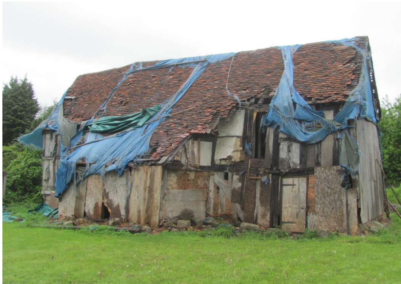
Photo of Master's House c 2017, showing inappropriate boarding and remains of tarpaulin
