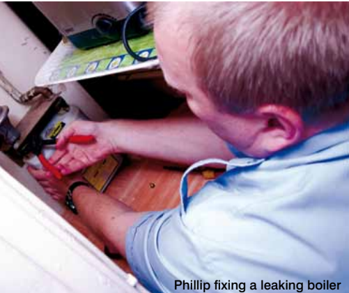
Phillip fixing a leaking boiler
